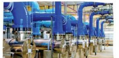
#3 UV LIGHT DISINFECTION AND ADVANCED OXIDATION
