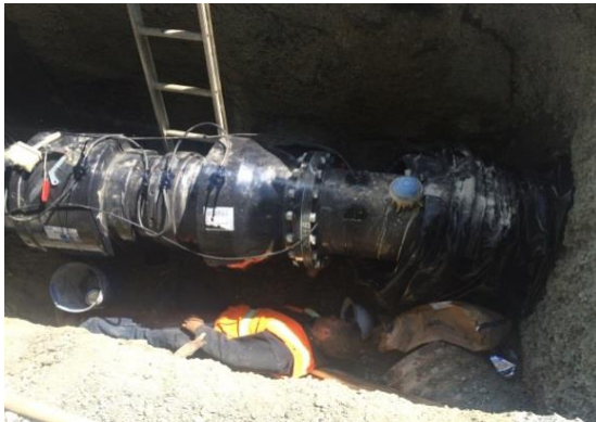
18-inch flexible expansion joint with ball marker on connecting ML&PCS pipe at Keith Avenue / Euclid Ave, Berkeley
