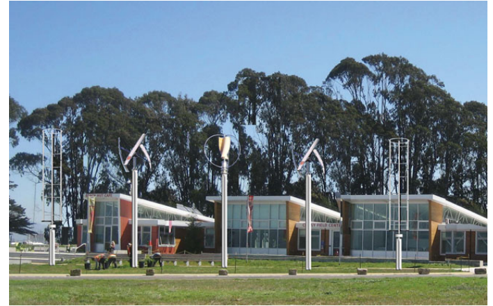
5 VAWTs totaling 6.8kW installed last month at NPS' Crissy Field Center
