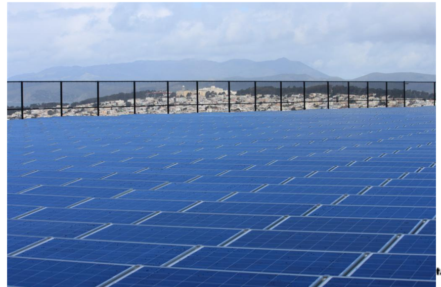
Sunset Reservoir – 5MW (2010)
