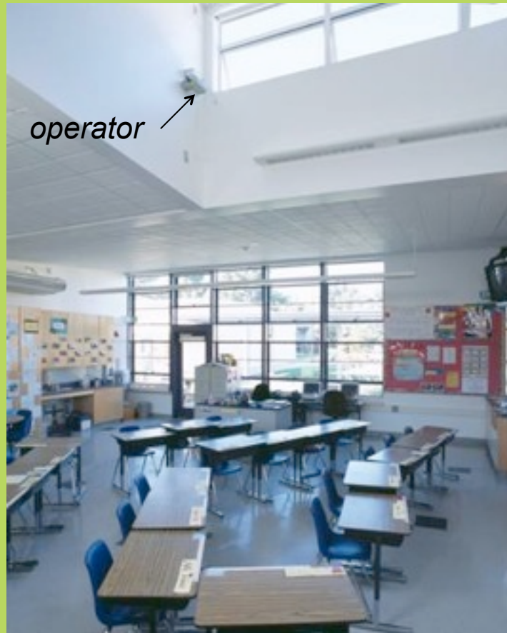
Energy management system activates clerestory window operator
