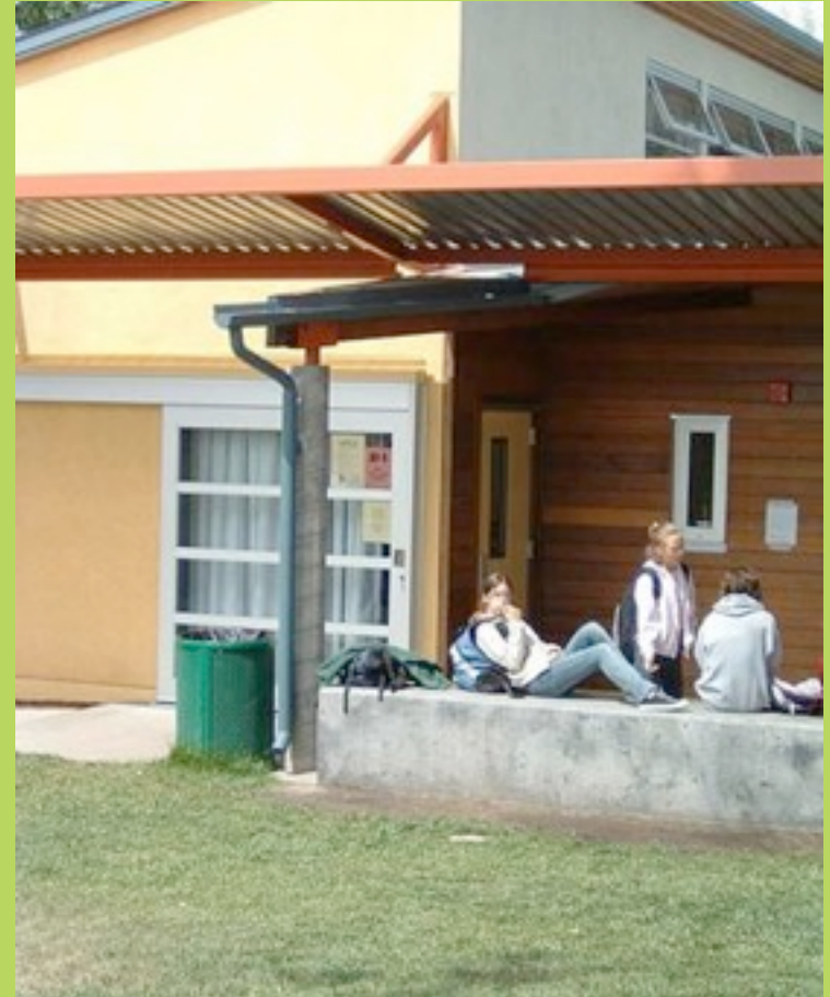
Roof run-off visible under canopy
