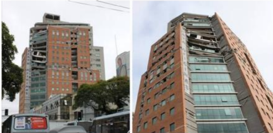
Apartment building, Concepcion; Photo courtesy of Jack Moehle, www.peer.berkeley.edu
