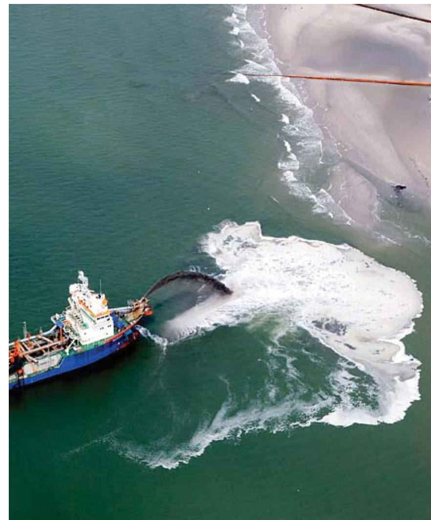
Beach nourishment, the deliberate placement of sand to counteract erosion, is a promising option at Ocean Beach, since 300,000 cubic yards of dredged sand from the Shipping Channel are available annually for beneficial local use.
