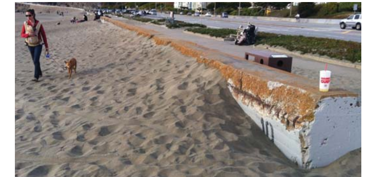
2012: Sand reaches the top of the seawall
